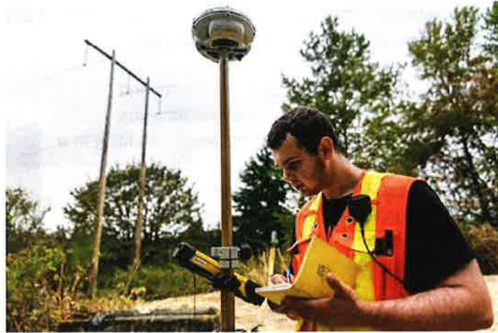
PSE contractor performs a land survey along the existing transmission line corridor in August 2015.
